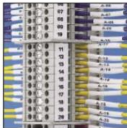
Terminal Block Labeling
