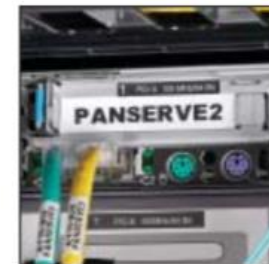
Network Infrastructure Labeling
