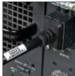
Electrical Infrastructure Labeling
