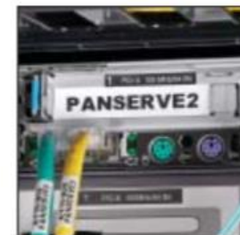
Network Infrastructure Labeling
