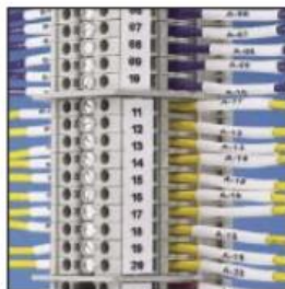
Terminal Block Labeling
