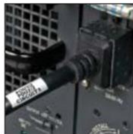
Electrical Infrastructure Labeling
