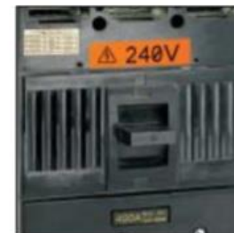
Electrical Hazard Labels
