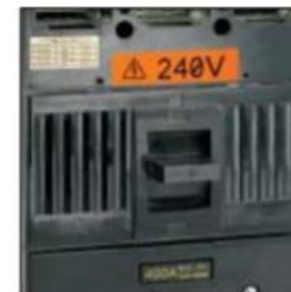
Electrical Hazard Labels
